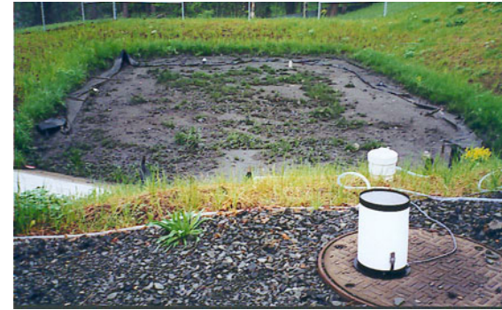
Surface Sand Filter
