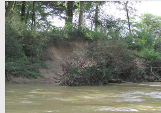
Figure 2.2-7 Chatahoochee River bank erosion caused by fallen tree undermined by scouring in high flows Photo: CRNRA, National Park Service, 9/5/15)
