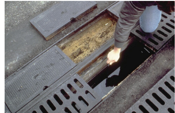
Perimeter Sand Filter
